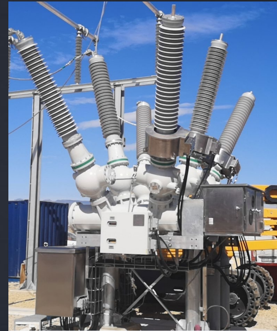
Hybrid Gas-Insulated Switchgear (HGIS)
